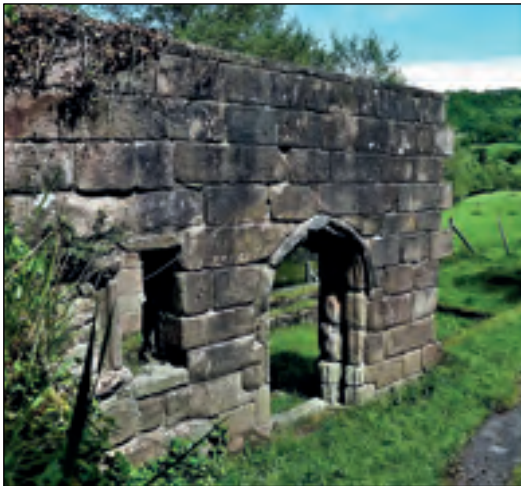
The south wall of the chapel, part of the structure that was rebuilt in 1951-1952, look-ing east towards the Meadows.
