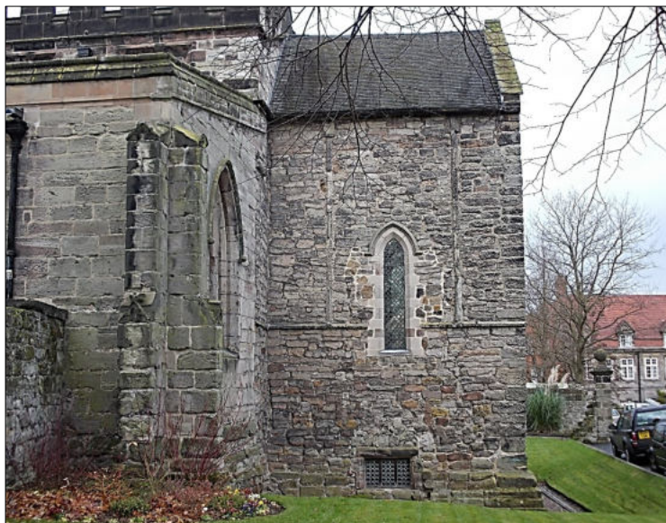
The east end of St Wystan's Church, with the Saxon chancel above the earlier crypt; note the typically Saxon strip pilasters flanking the later Early English window.
