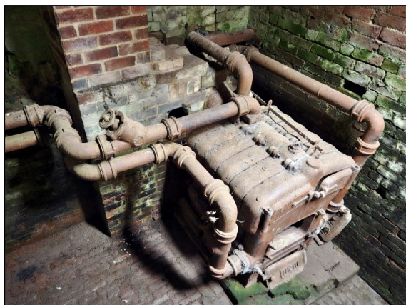
A 'Robin Hood' boiler manufactured by the Beeston Boiler Company, installed underground to provide greenhouse heating in the gardens at Calke Abbey.
